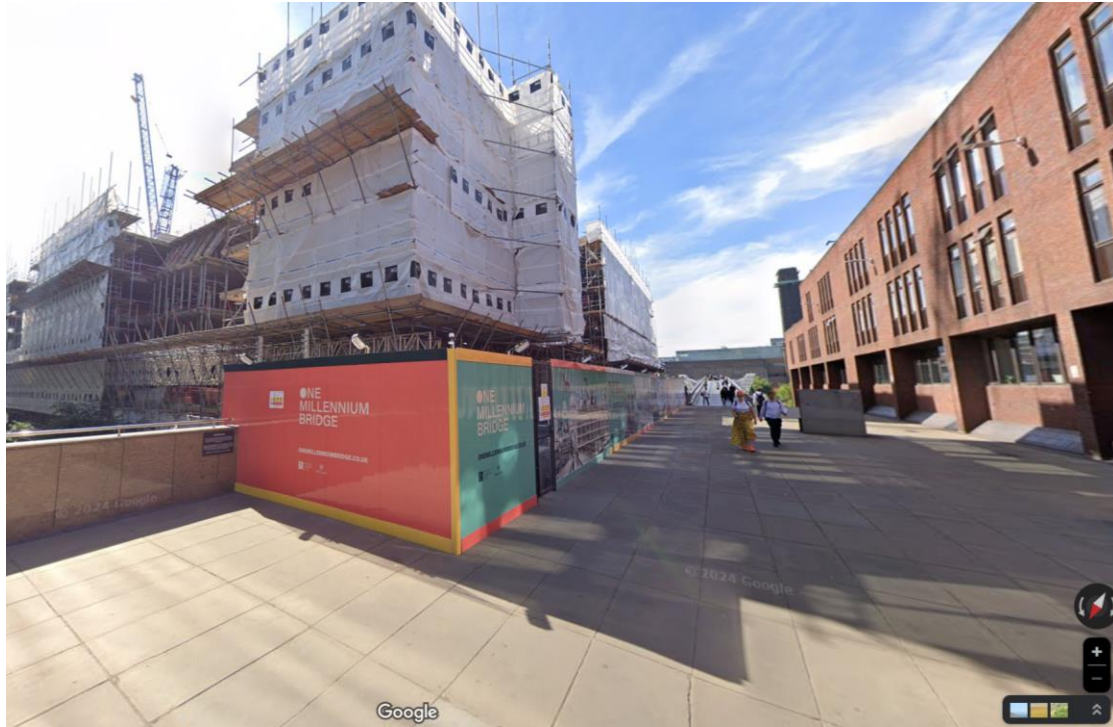
Existing | Millennium Bridge House under construction, looking south to the Bridge (circa June 2022)
